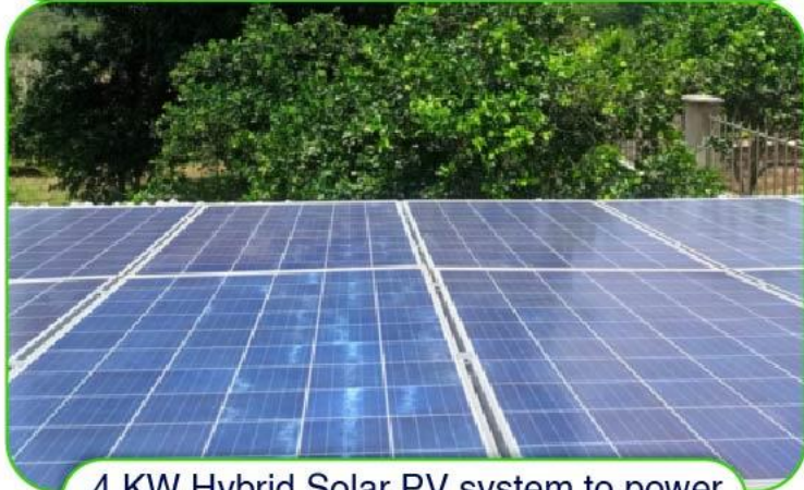
4 KW Hybrid Solar PV system to power a 4 bedroomed residential house in Shimba Hills.
