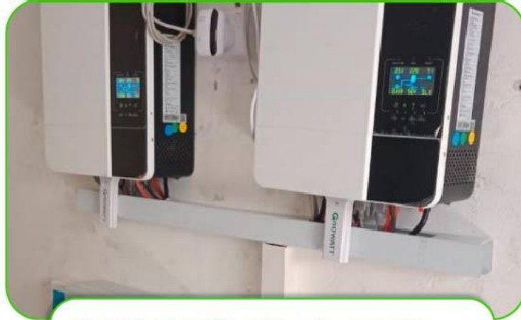
10 KW solar PV system to power a hotel in Malindi
