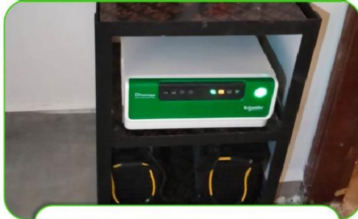
1.5 KW solar PV to power a 3 bedroomed residential house in Vipingo
