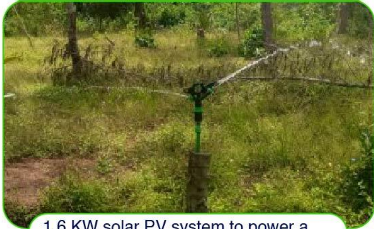
1.6 KW solar PV system to power a farm & pump water for home use & irrigation in Ramisi.
